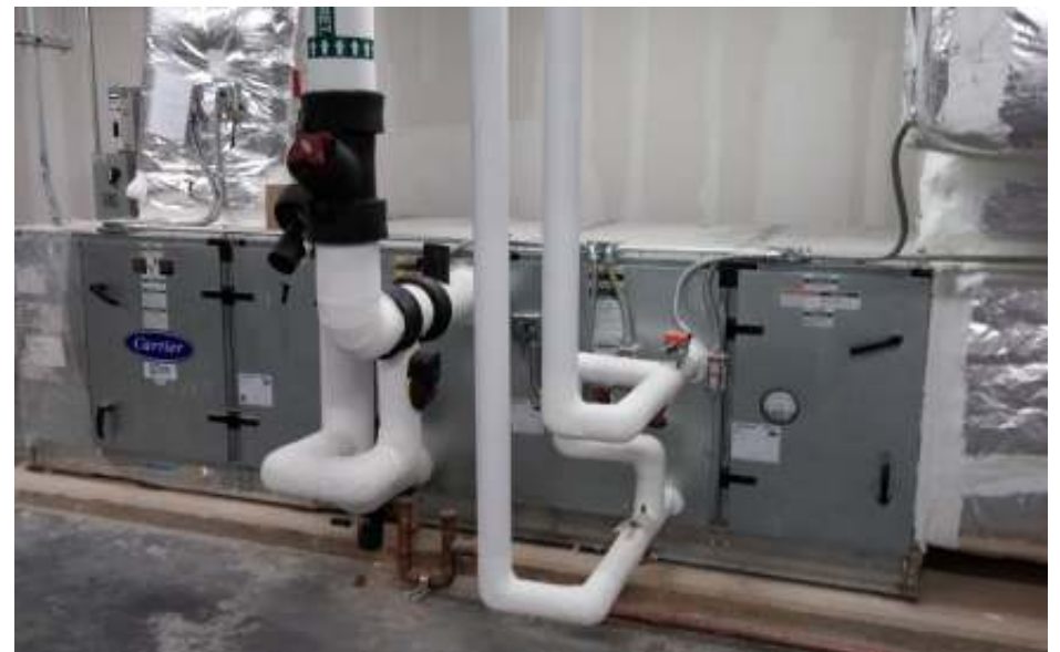
Chilled water, hot water & duct insulation at an Air Handling Unit in the mezzanine servicing the ticket area.
